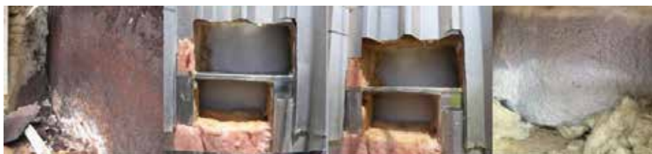
Figure 9: IMM coating in CUI mitigation service: original corroded condition (left), 5 and 13 years (middle), and 20 years (right)
